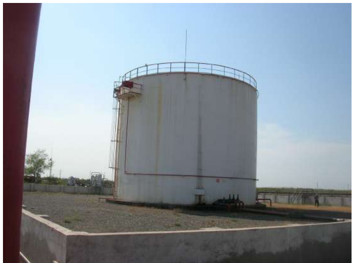
3000 BBL Oil Storage Tank at Muradkhanli Central Facilities
