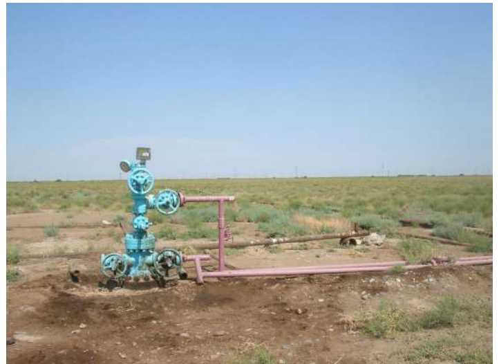
Typical Flowing Muradkhanli Oil Well
