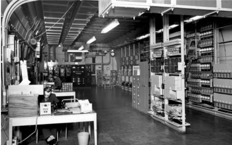
From 1949 onwards, the tunnels began to be used as a secure and secret long-distance telephone exchange. DBOX/The London Tunnels
